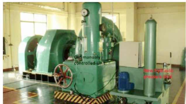
The turbine and generator and manually operated hydraulic control valve, next to a new electronically operated hydraulic control valve
