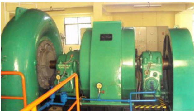
The turbine and generator
