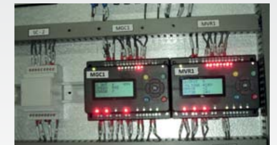
MIACs used to control a mid scale hydroelectric power station in Sri Lanka.
